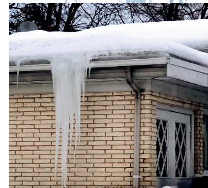
Large icicles have the potential to cause extensive damage and serious injury. PHOTO COURTESY OF MICHAEL HUSTON, LINDHOLM ROOFING, CHICAGO, ILLINOIS.
