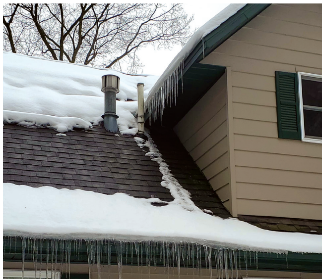
The lack of snow in the roof plain shows where heat is transferring from the conditioned living space to the attic, indicating inadequate insulation and/or inadequate ventilation. PHOTO COURTESY OF TIM CHAPIN, YOUR SAFE AND HEALTHY HOME, AKRON, OHIO.
